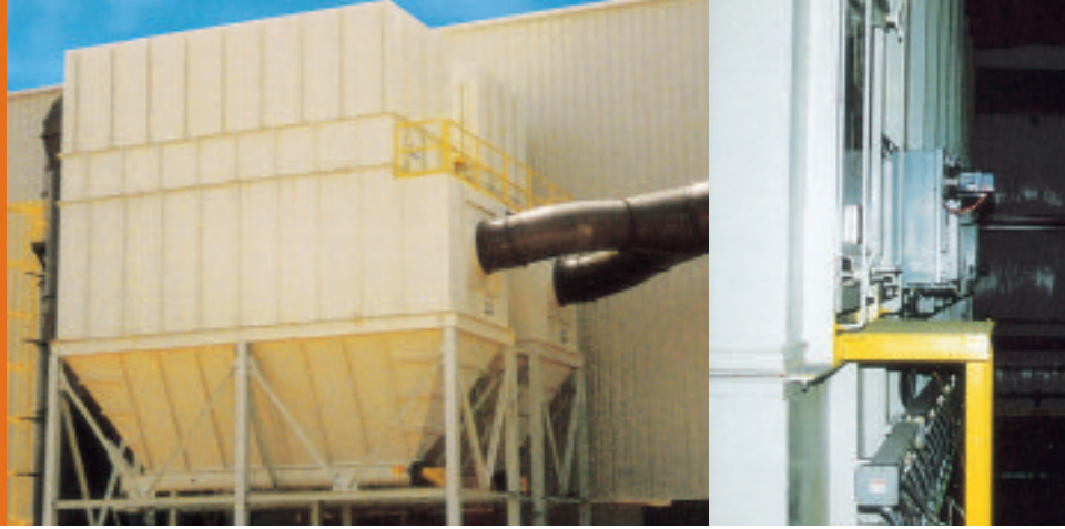
(2) Model 1538-10 Dust Collectors on Foundry Melt System
