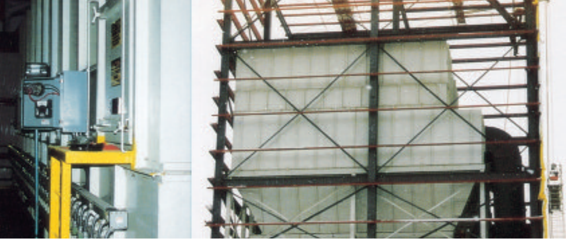
(2) Model 1550-10 Collectors in Sand Tower of Foundry Sand System
